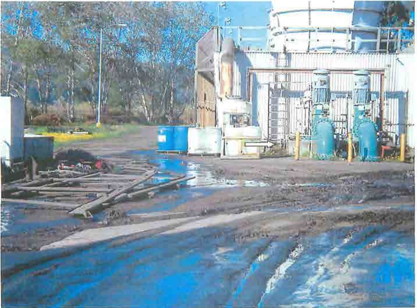
Photograph 6. Ash and slurry from the site. Barrels containing chemicals are present without proper secondary containment.
