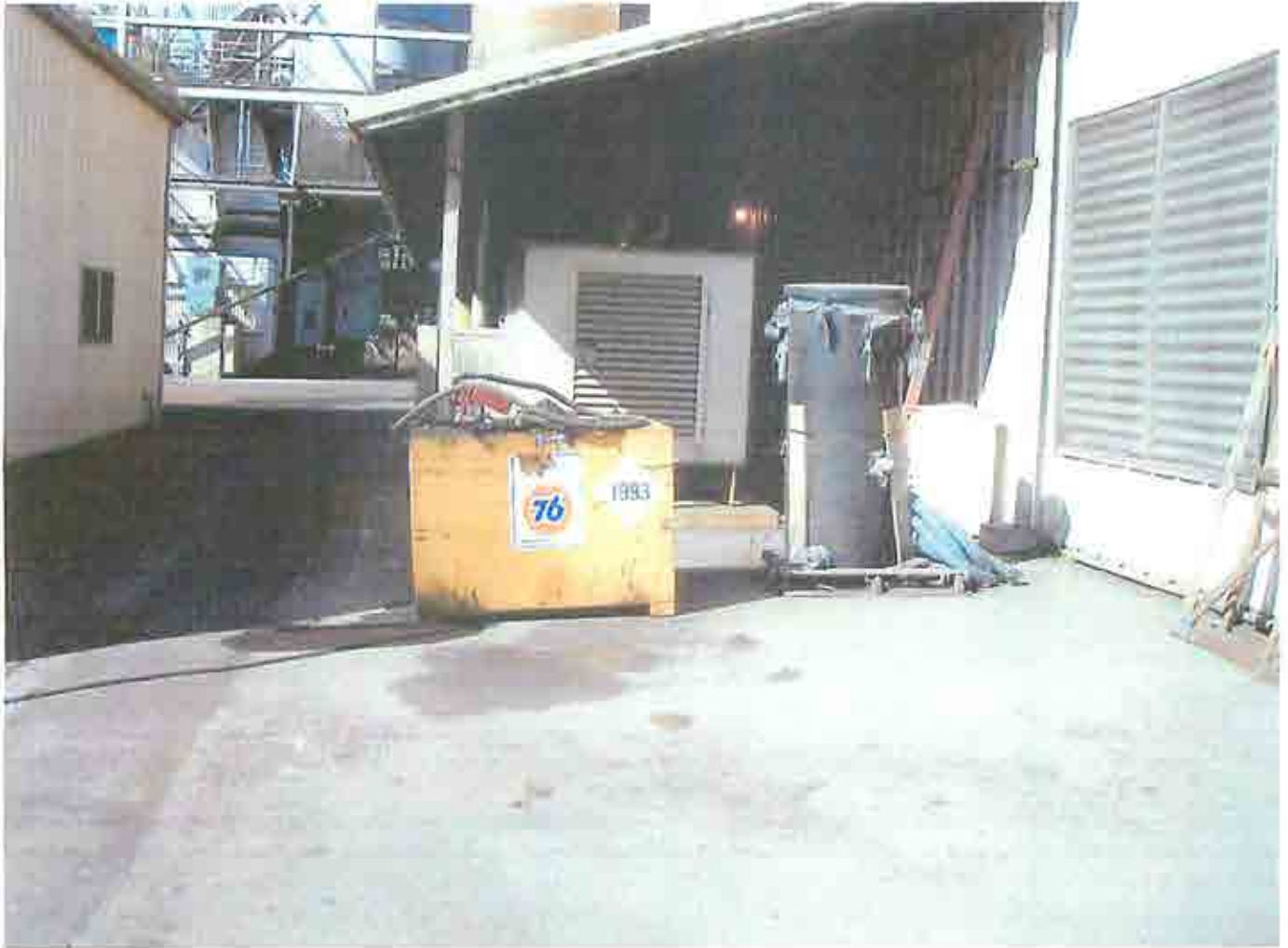
Photograph 7. Diesel fuel onsite without secondary spill containment measures.
