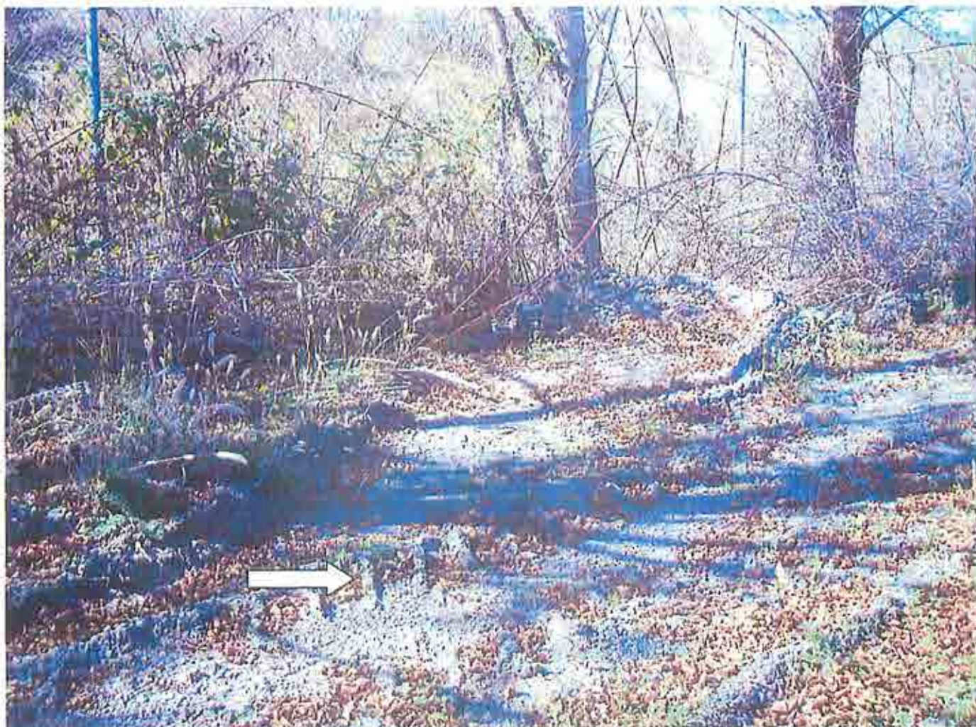
Photograph 5. Equipment tracks (arrow) left from apparent breaching of straw wattles. Straw wattles were intact in other areas of the site, however, at this point, they appeared to have been removed and runoff directed toward the tributary to the Mad River.
